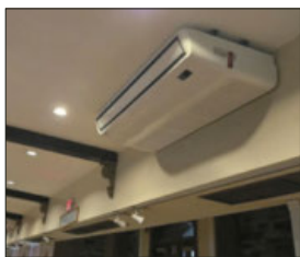
Updated Air Conditioning Units at St. Joseph's Chapel
